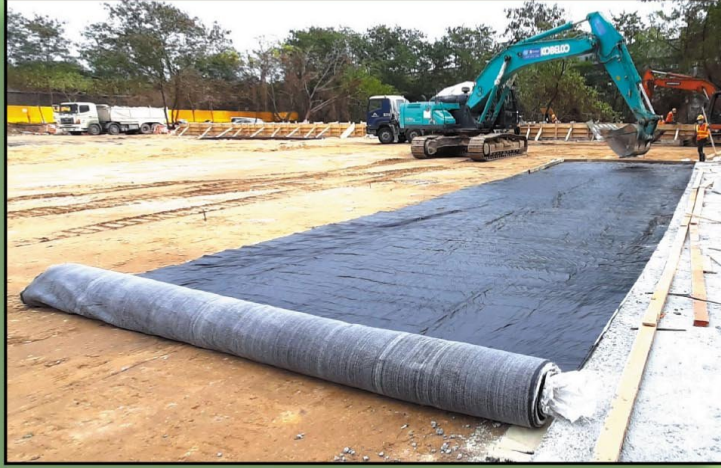
Lok Ma Chau Loop (YL/2020/02) GCL Wetland Waterproofing, January 2022 落馬洲河套區濕地防水粘土襯墊
