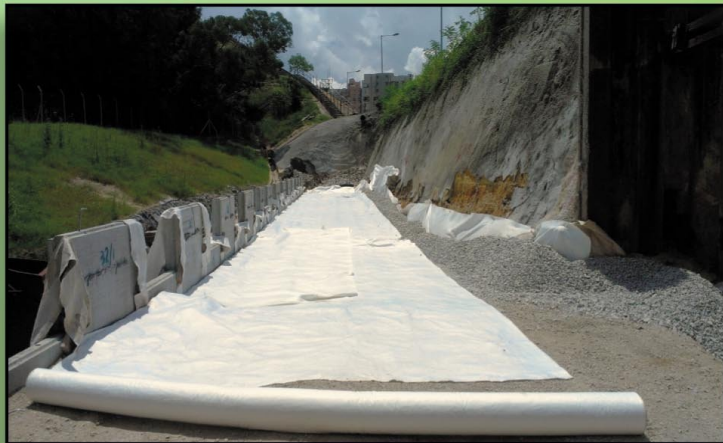
Tuen Mun Road (HY/2008/11) Geotextile Drainage Separation, August 2012 屯門公路重建分隔土工布
