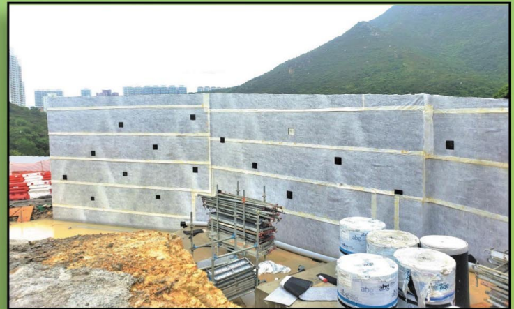
Tung Chung New Town (NL/2020/02) Geocomposite Retaining Wall Drainage, August 2022 東涌新市鎮擋土牆排水板
