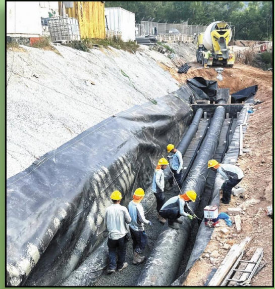
Fresh Water Service Reservoir (2/WSD/20), HDPE Geomembrane Leakage Collection, January 2024 食水配水庫防漏及收集土工膜
