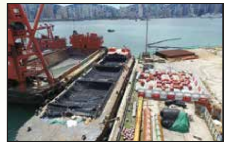
Geotextile container for contamination disposal, SCL cross harbor tunnel, Jan 2015 沙中線海底隧道污染泥處理土工布袋
