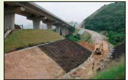
Erosion control mat stays intact after 20 years, Tsing Yi Northern Coastal Road, Sept 1999 青衣北路防侵蝕墊安裝20年後仍維持完整
