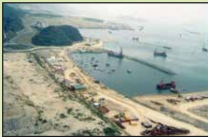
Woven geotextile, sand layer separation along seabed, TKO Reclamation, Jan 1993 將軍澳填海織土工布穩定海床及分隔沙塵
