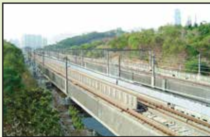
Recapping disused landfill for Airport Express Viaduct to pass through, Gin Drinkers' Bay, Apr 2005 機場快線葵涌公園繞道，醉酒灣舊垃圾堆填區封頂
