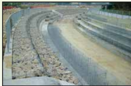
Ecology enhancement with Gabion, Tai Kong Po River Channel Rehabilitation, Kam Tin, Nov 2004 大江埔生態石籠
