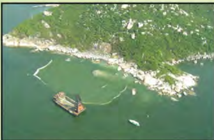
Silt curtain, CLP Cable Tunnel, Tai Long Wan Landing, July 2003 芝蔴灣至大浪灣電纜隧道海岸隔泥幕
