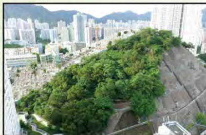
Geocell supported slope vegetation, Tung Tau Cottage, Sept 2002 東頭邨土工格室支撐邊坡植物樹木
