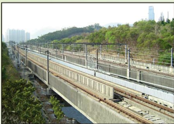
Recapping disused landfill for Airport Express Viaduct to pass through, Gin Drinkers' Bay, Apr 2005
