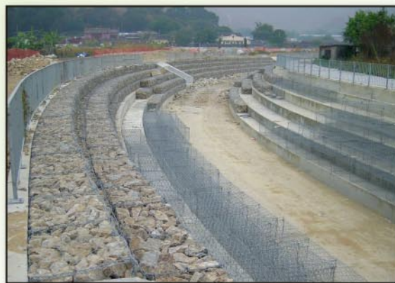
Ecology enhancement with Gabion, Tai Kong Po River Channel Rehabilitation, Kam Tin, Nov 2004
