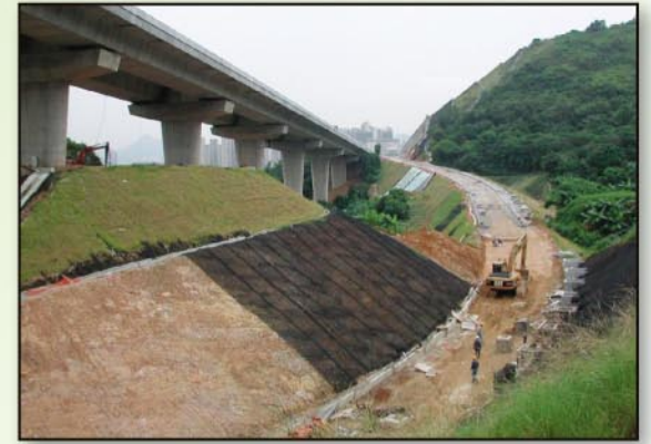
Erosion control mat stays intact after 20 years, Tsing Yi Northern Coastal Road, Sept 1999
