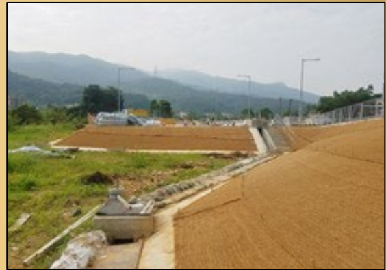
Access Road joining She Shan Road, Tai Po, and Improvement of Nam Wai Road, Sai Kung, November 2018 (HY/2014/13)
